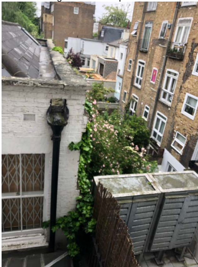
Two Extraction ducts at the rear of 84 Westbourne Grove:
